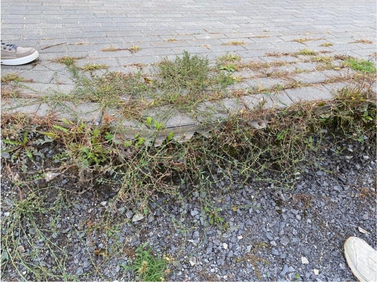
Figure 36: Photo of the overgrown vegetation in cracks of pathway at Site #1.
