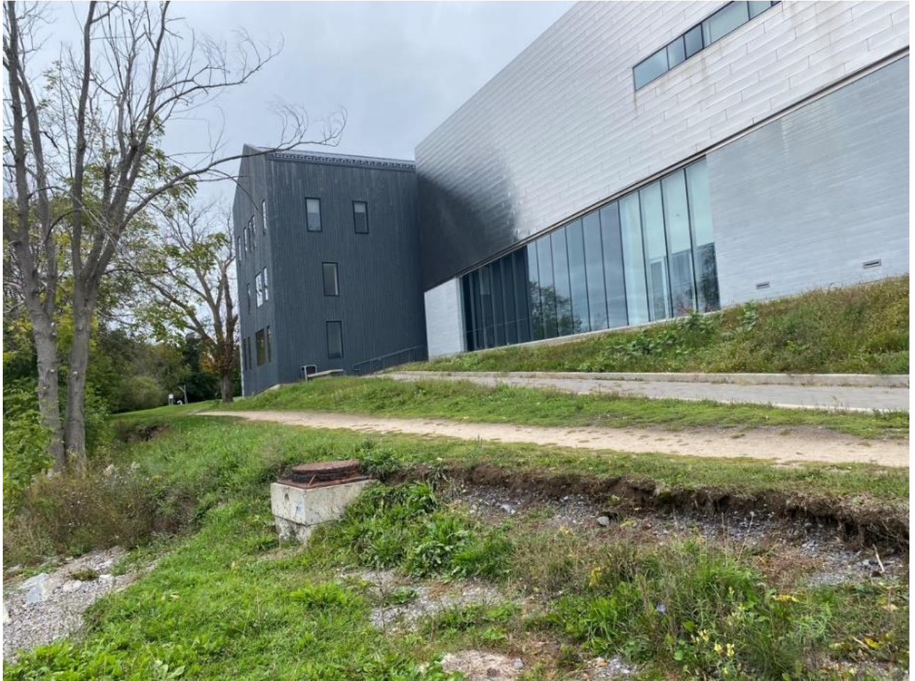
Figure 35: Photo of the eroding soil above the retaining wall at Site #1.
