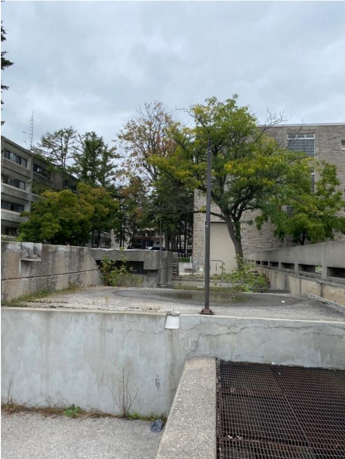
Figure 38: Photo of the concrete area and ventilation grate West of Jeffery Hall at Site #2.
