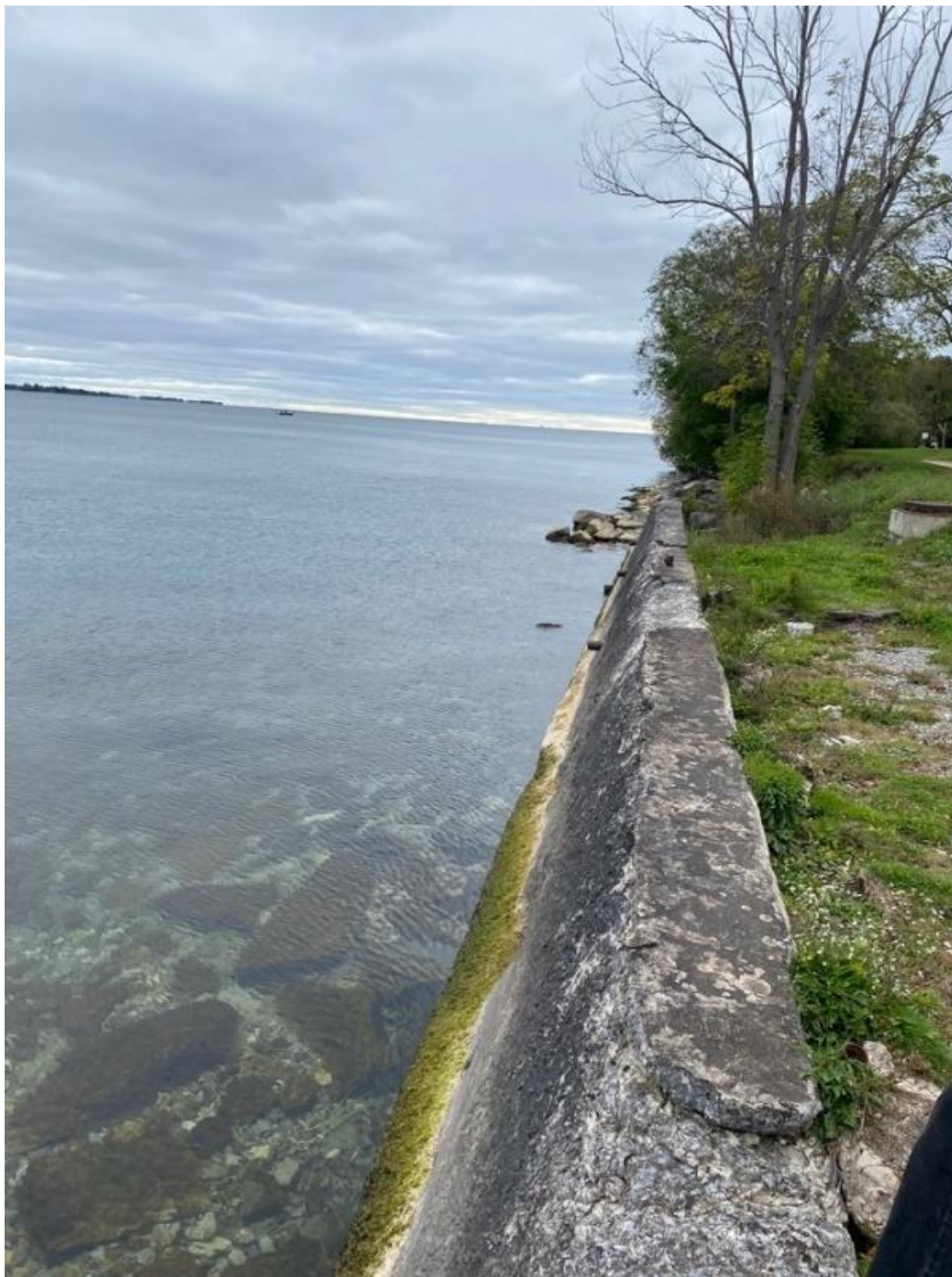
Figure 31: Photo of the deteriorating retaining wall with extruding pipes at Site #1.
