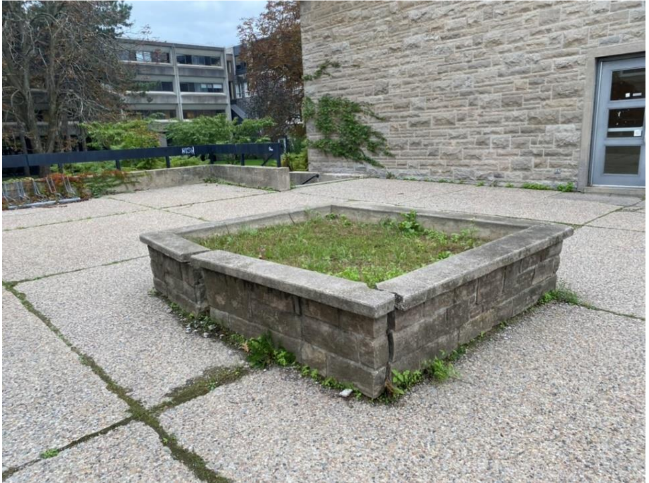
Figure 55: Photo of one of the cracked planter boxes at Site #5.
