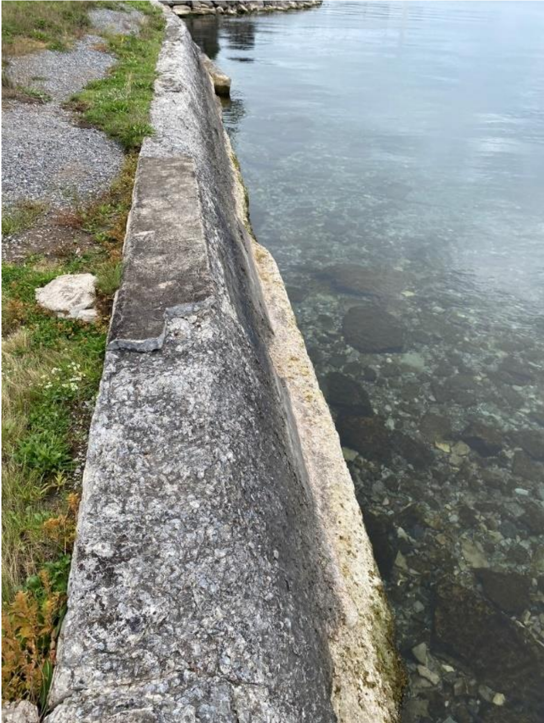
Figure 32: Another photo of the degrading retaining wall at Site #1.
