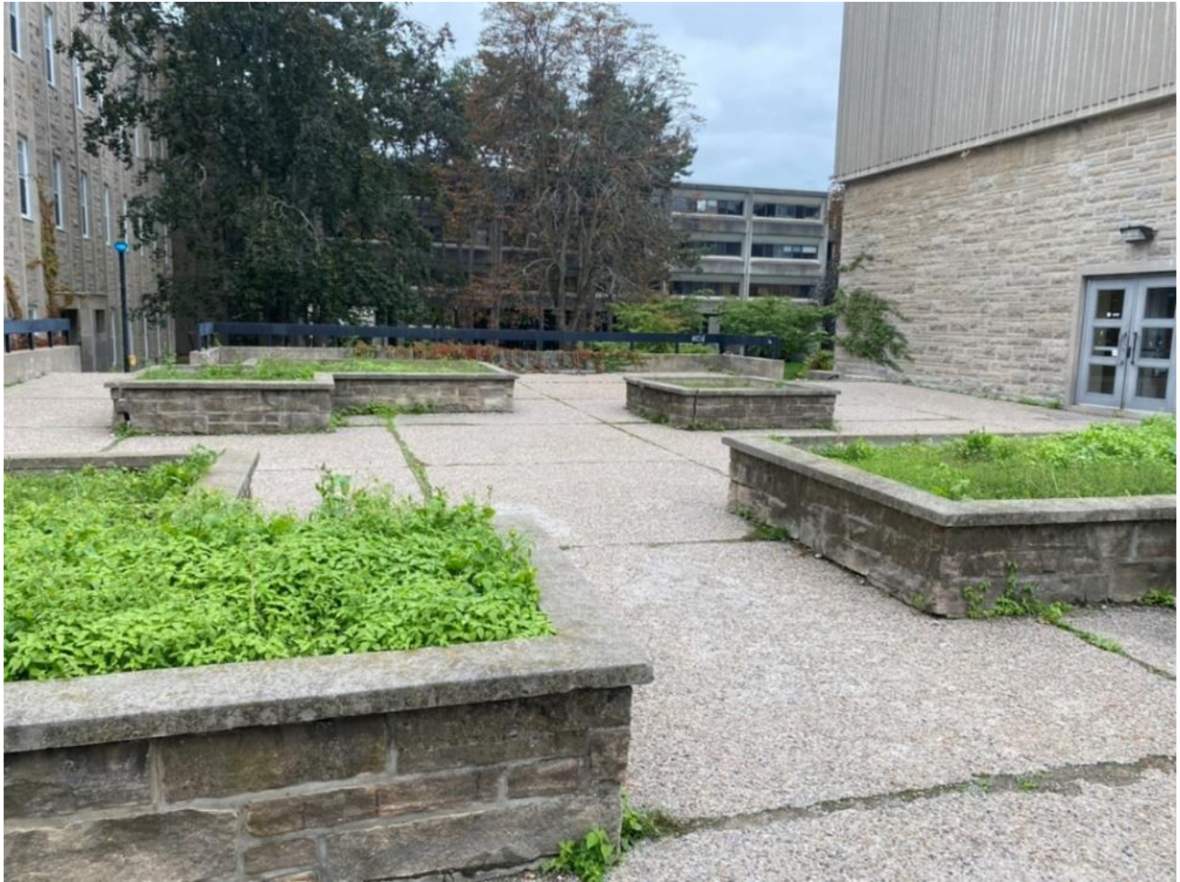
Figure 54: Photo of the planter boxes at the East side of the Queen's Law Building (Site #5).
