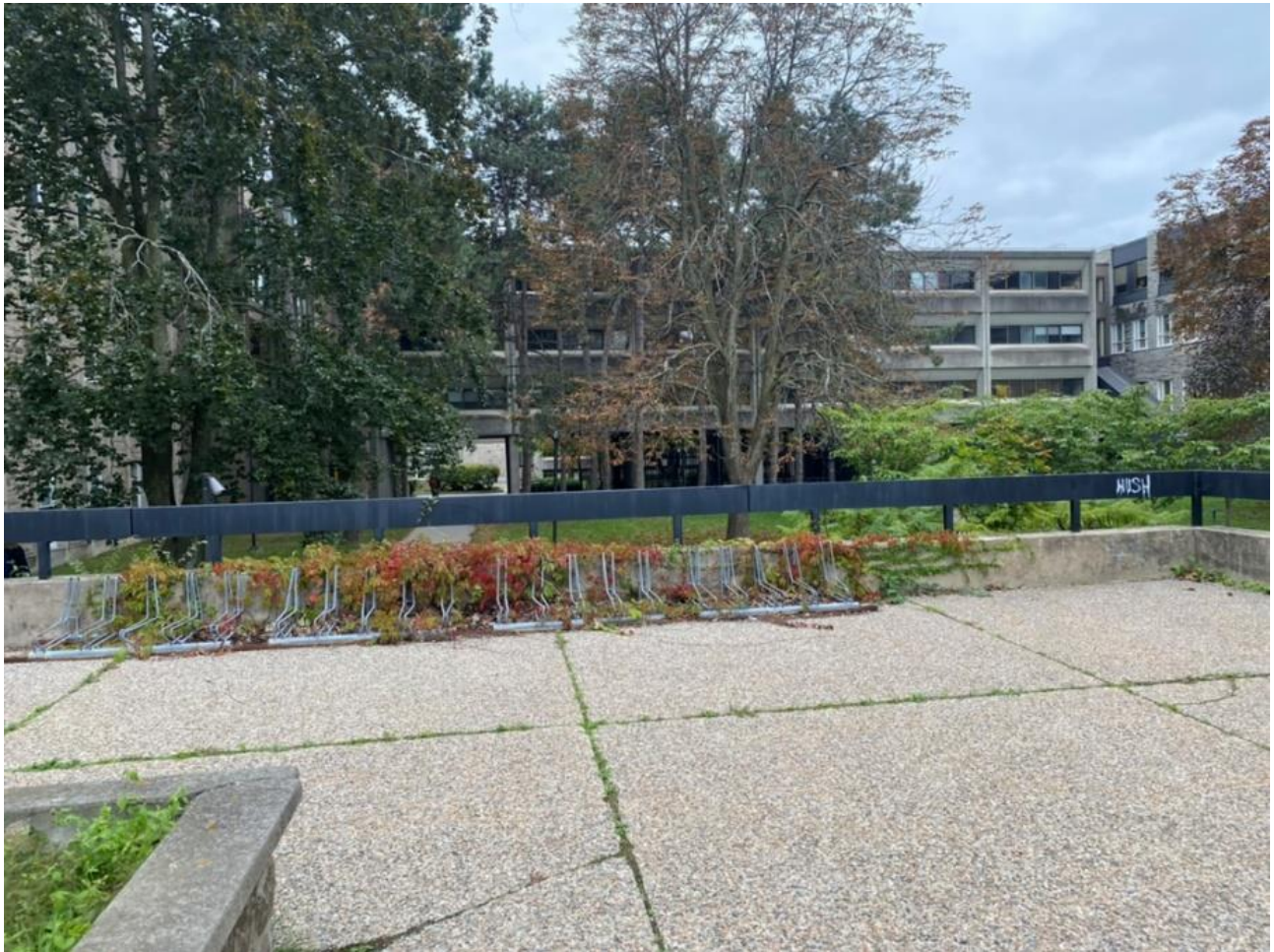
Figure 56: Photo of the cracked concrete South of the planter boxes at Site #5.
