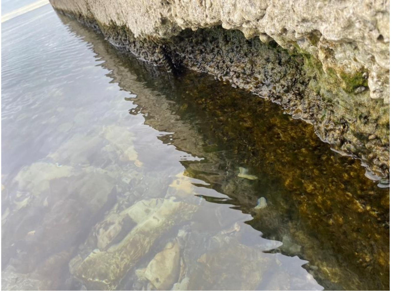
Figure 34: Close-up photo of the deterioration of the retaining wall concrete at water level at Site #1.
