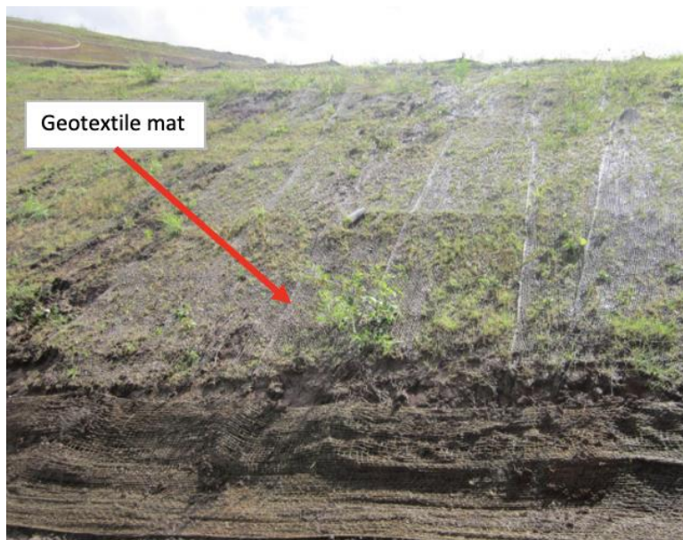
Figure 13: Geotextile mat used to control erosion on a steep slope (United States Environmental Protection Agency 2021).
