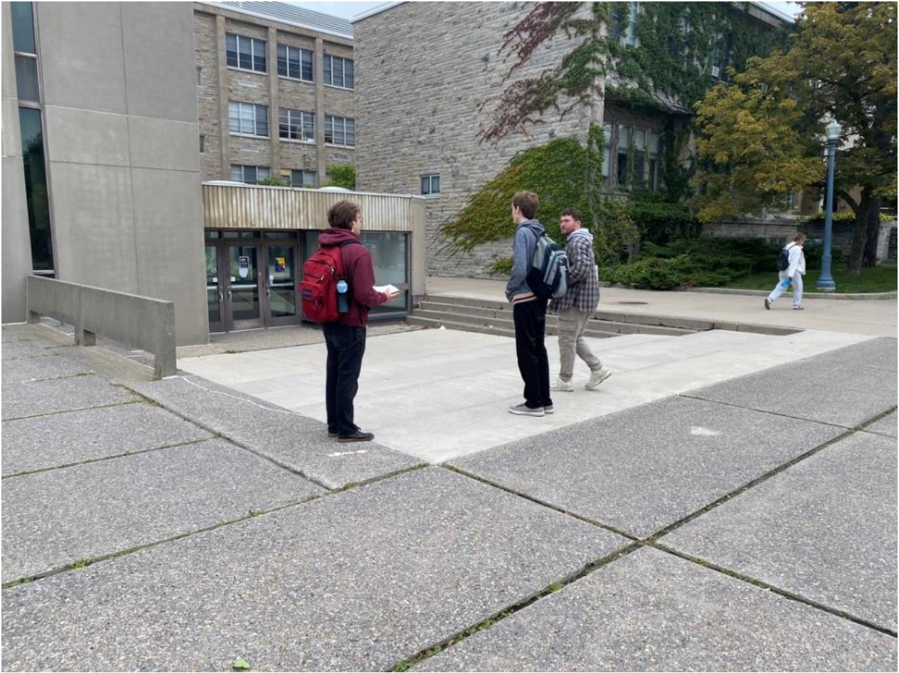
Figure 47: Photo of the large concrete steps at the East entrance of Jeffery Hall (Site #3).
