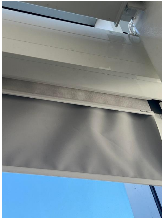
Figure 6: Existing Fully Automated Double-Blind System at Mitchell Hall.
