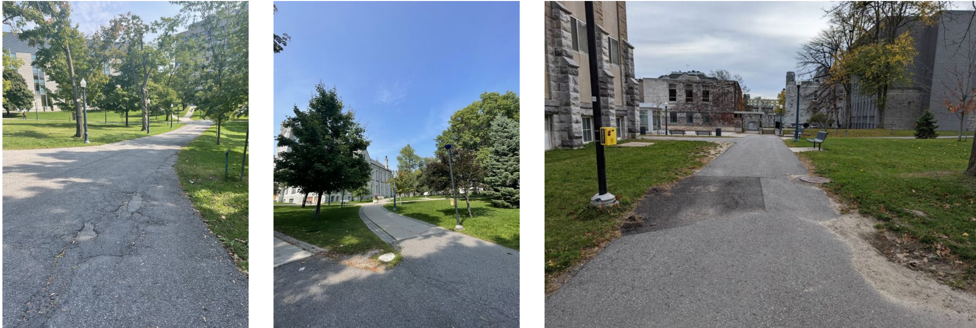
Figure 4-2 (Left): Poor material quality along the Summerhill driveway. (Middle): Inconsistent pathway materials present between Summerhill and Theological Hall. (Right): Poor material quality and selection along the pathway west of Nicol Hall.
