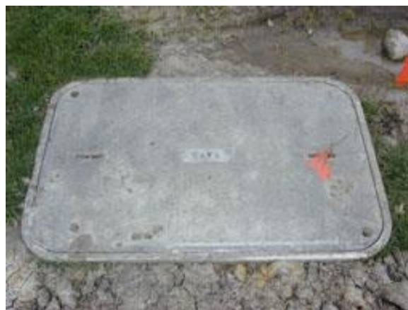
Figure 4: Fibre Optic Access Hatch (Purdue University 2000)
