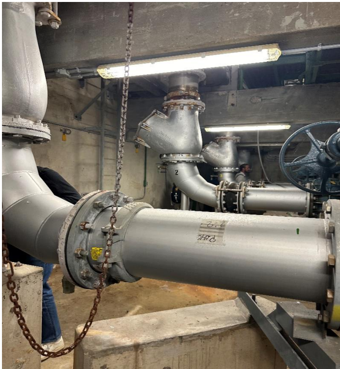
Figure 15: Various pipeline systems of wastewater in Wastewater Pumping Station
