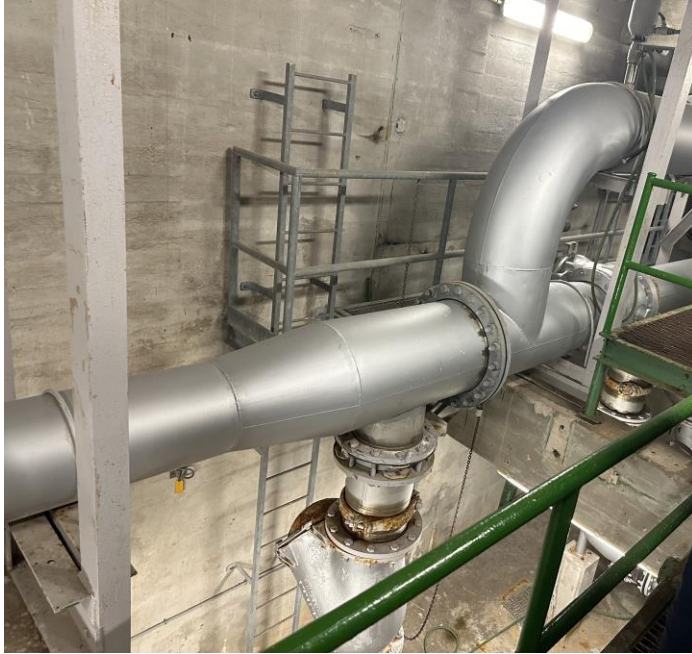
Figure 14: Junction of pipes in Wastewater Pumping Station on Queen's University Campus
