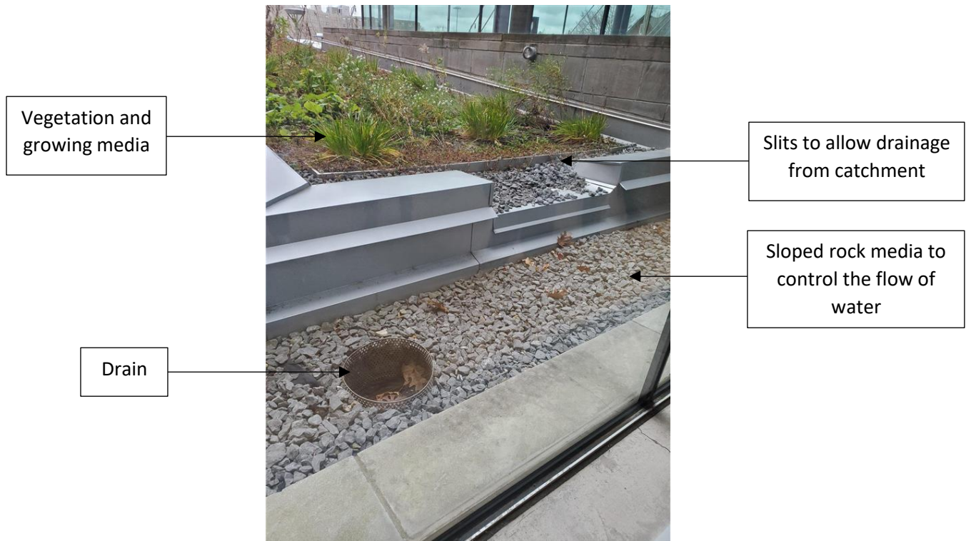
Figure 15: Goodes Hall green roof drainage system. Photograph taken 13/11/20.
