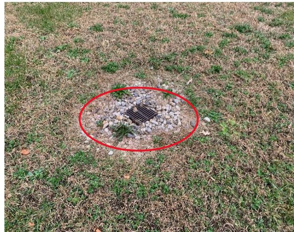
Figure 11: Drainage system on Biosciences green roof; image taken by Greengenuity (11/13/2020).
