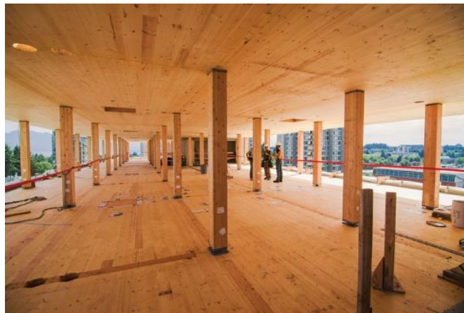
FIGURE 8: COLUMN AND TWO-WAY CLT PANEL SYSTEM IN THE BROCK COMMONS BUILDING (BROCK COMMONS)
